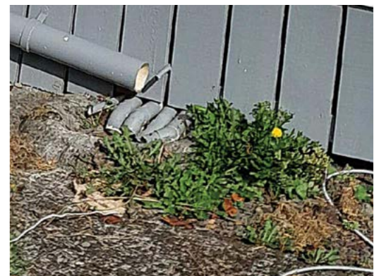
Two examples of non-compliant gully traps
