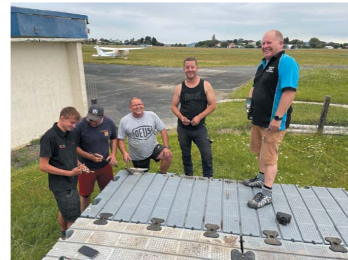
Building the pontoon - All fire volunteers, From left - Cameron Jones, James Restall, Jeff Pipe, Justin Rankin and Brian Redwood
